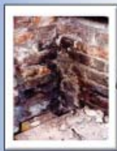
Below is a deteriorated chimney, which caused the flue to be blocked
